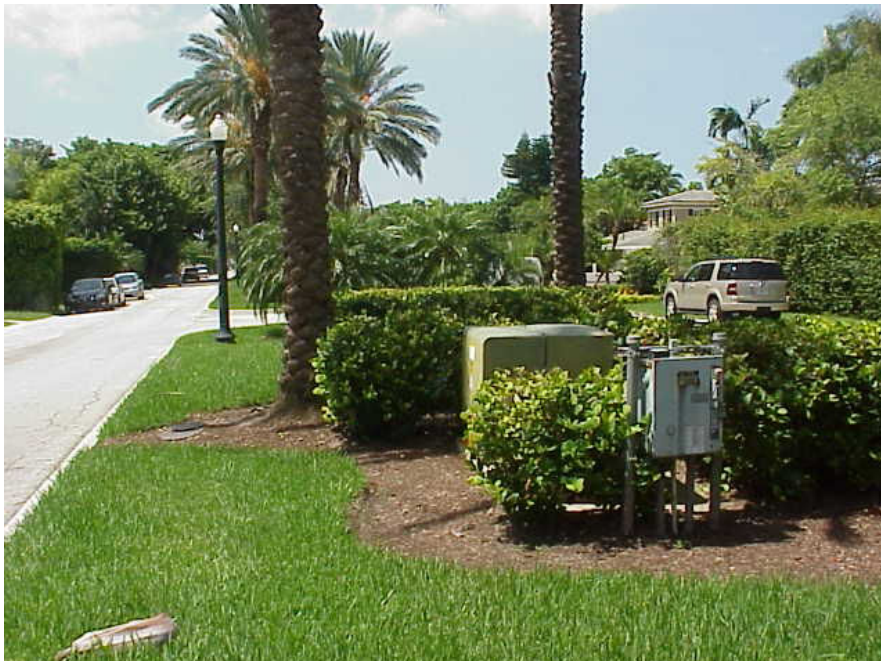
Figure 3-3. Underground equipment in the median of Allison Island.
