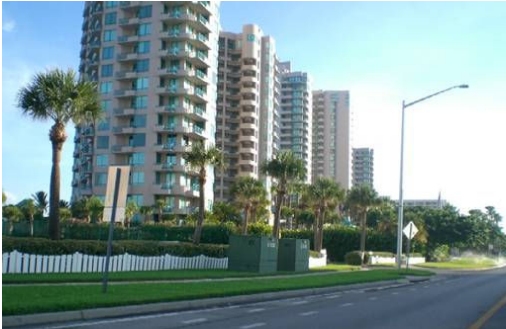
Figure 4-4. Pad Mounted Equipment on the Side of the Road in Sand Key
