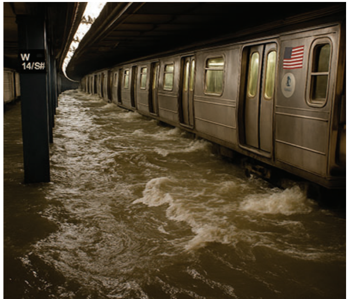
Flooding caused by Hurricane Sandy inundated not only the NYC subway system, but also Con Edison's underground electrical substations, leaving at least 220,000 customers without power for an extended period. The substation repair bill exceeded $561 million ($790 million in 2025 dollars).
