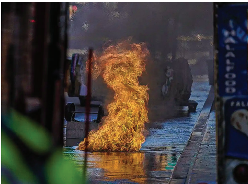
Caused when highly flammable gases accumulate in underground vaults and are ignited by sparks from an arc, “manhole events” include explosions powerful enough to blast manhole covers several stories into the air. Nearly all such events are associated with buried electrical systems. To view a short video of a few very-near misses visit https://bit.ly/manhole_events .
