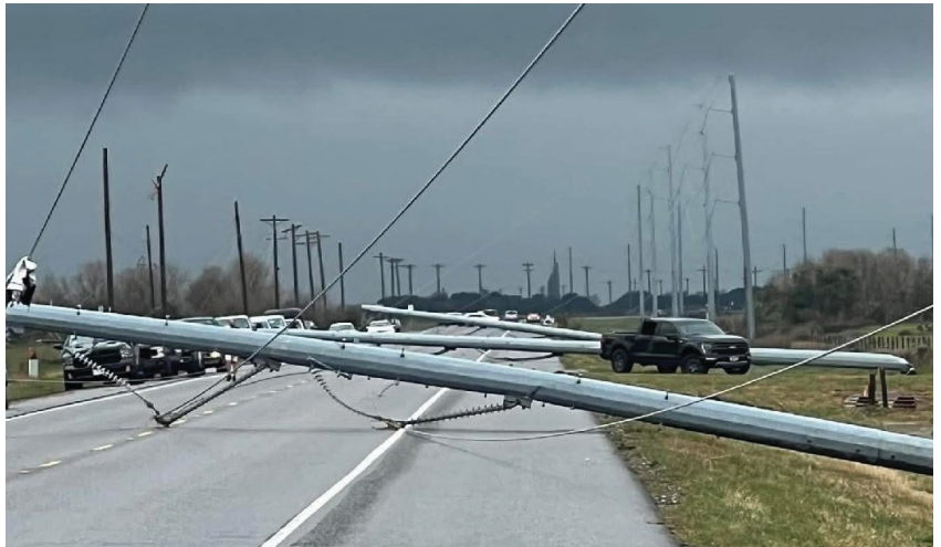
These steel poles collapsed when an tornado with 161 mph winds hit southeast Texas in late December 2024. The still-standing wood poles in the background survived due to wood's wide coefficient of variance allowing them to withstand forces beyond their assigned design capacity.
