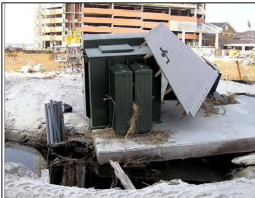
Figure 6: Destruction of Pad-Mounted Transformer Caused by Tidal Surge And Beach Erosion from Hurricane Ivan (2004)
