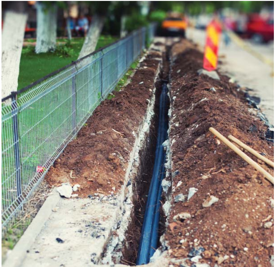
Figure 1 - Moving overhead lines underground is not only expensive, but creates significant disruptions in the areas where such work is done. Most undergrounding conversion projects require cutting through concrete or asphalt, forcing detours for traffic and pedestrians. Excavating also may be necessary to make repairs in underground systems should there be power failures.
