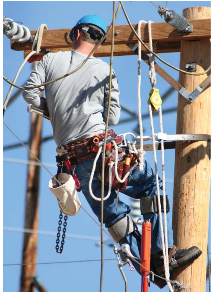
Figure 1 - Unlike underground systems, most repairs to electrical service can be done by linemen who have the appropriate gear to restore service quickly and economically.
