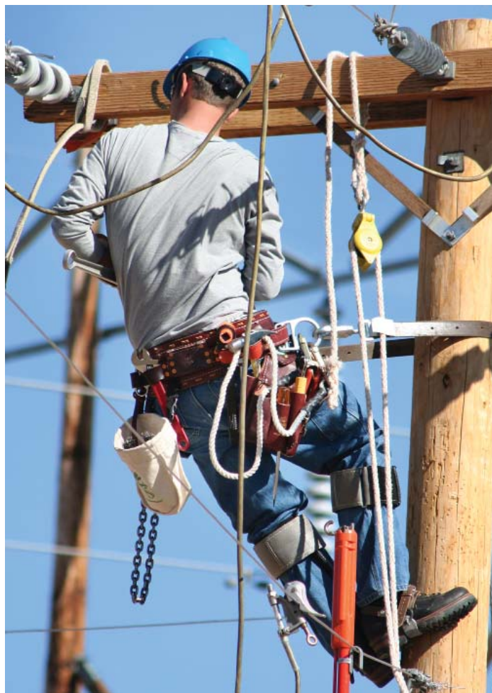
Figure 1 - Unlike underground systems, most repairs to electrical service can be done by linemen who have the appropriate gear to restore service quickly and economically.
