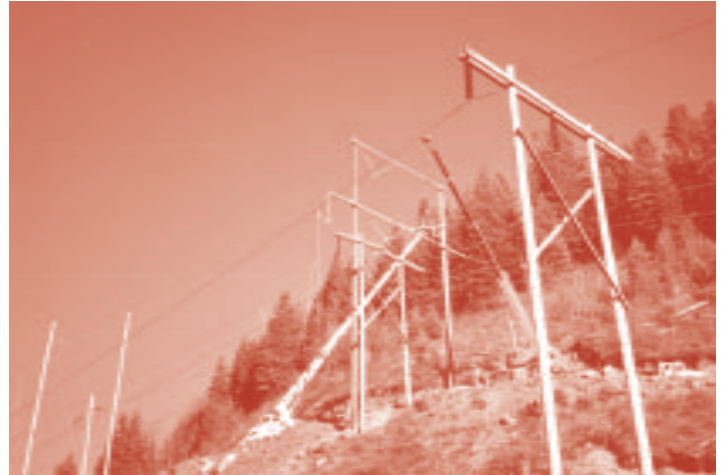
An existing 230kV circuit is relocated from one of the wood H-frame lines to the new double circuit H-frame.
