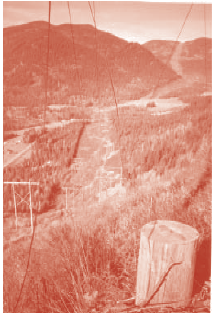
To accommodate a narrow rugged right-of-way, a BC Hydro 230 KV circuit is relocated from an existing wood H-frame structure to a new double circuit H-frame structure.
