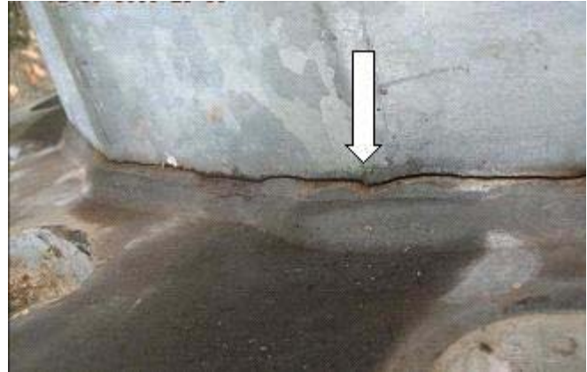
Close-up - crack near weld that joins the pole to its base plate
