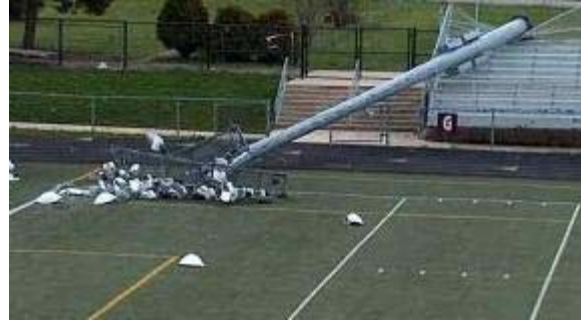
Fallen stadium light poles
