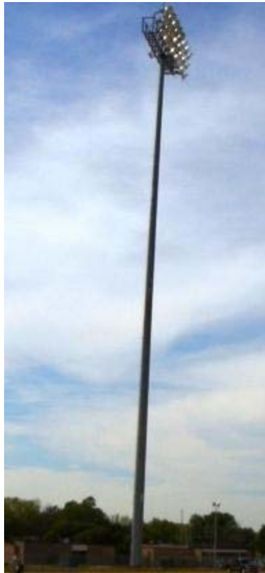
Upright stadium light pole
