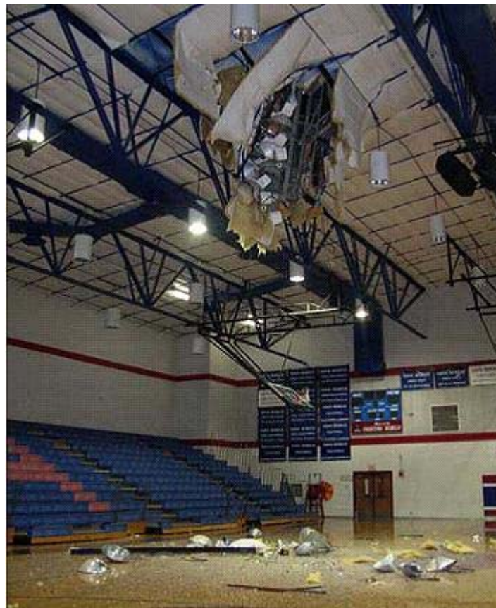
Stadium light pole fallen through gymnasium roof
